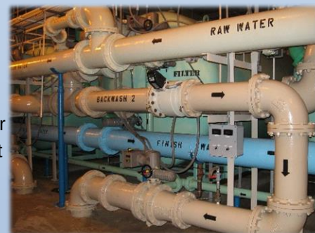
Filter Room at the Charles River Water Treatment Facility
