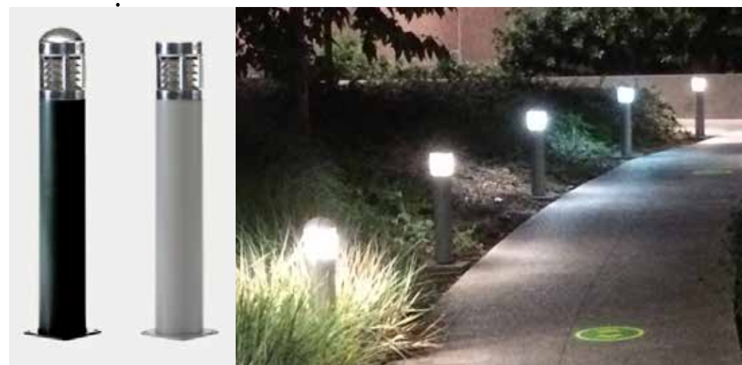
Bollard Lights at HC Parking
