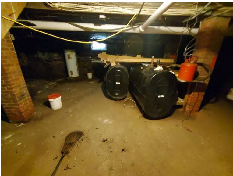
Photo #9: Two ~275 gallon fuel oil tanks located in the basement
