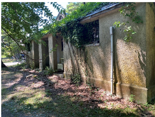
Garage Electrical Service
