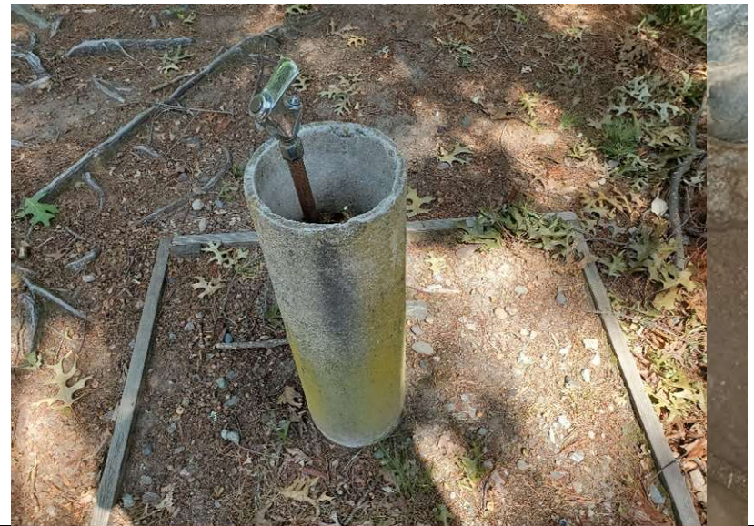
Photo #20: A water fountain containing asbestos
