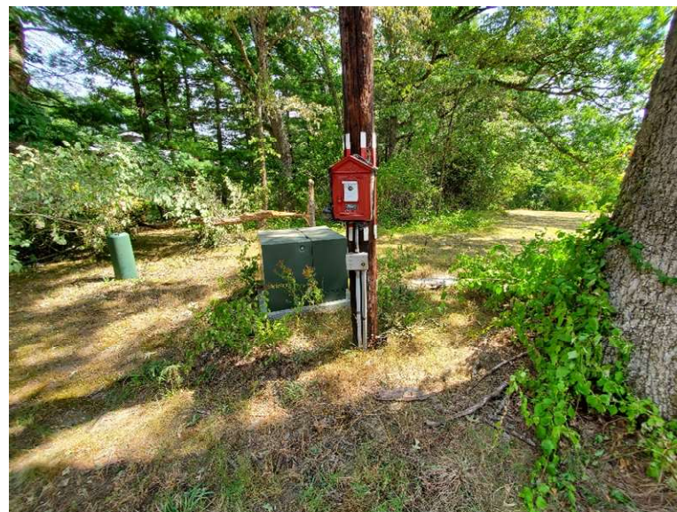
Photo #2: Transformer located in front of the manor house
