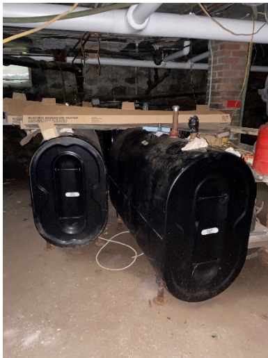
Estate House Oil Storage Tanks – Basement
