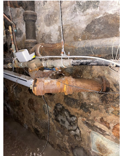
Water meter Ridge Hill Estate House
