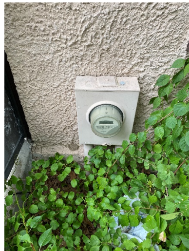
Estate House Electric Meter
