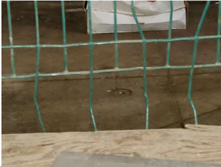
Photo #17: Cleanout system located in the garage
