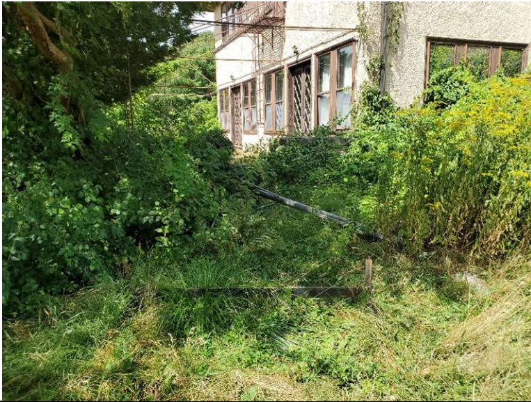
Photo #5: Overgrown area of the exterior of the manor house
