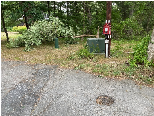
Transformer, Telecommunications Pedestal & Master Box
