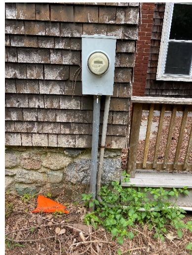
Barn/Ranger's Residence Electric Meter
