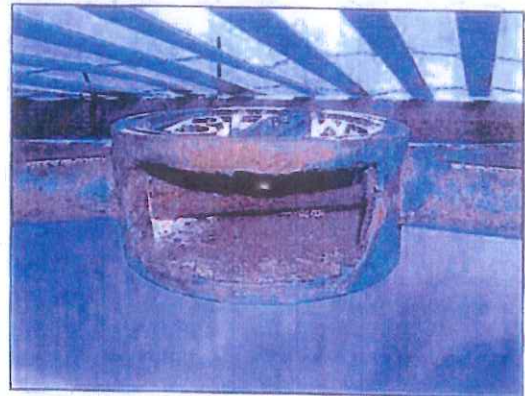
Cast Iron Spalling at Rosette
