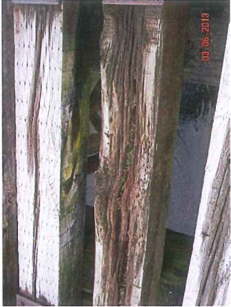
Figure 53: Deteriorated Timber Ties
