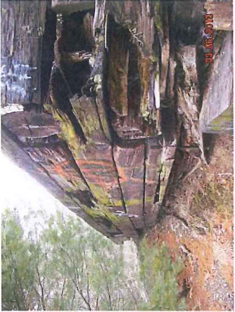
Figure 54: Deteriorated Northwest Abutment
