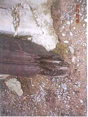
Figure 55: Deteriorated Timber Pile and Soil Erosion at Abutment
