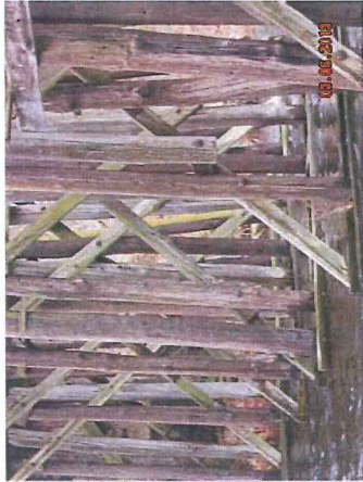
Figure 52: Missing Timber Piles
