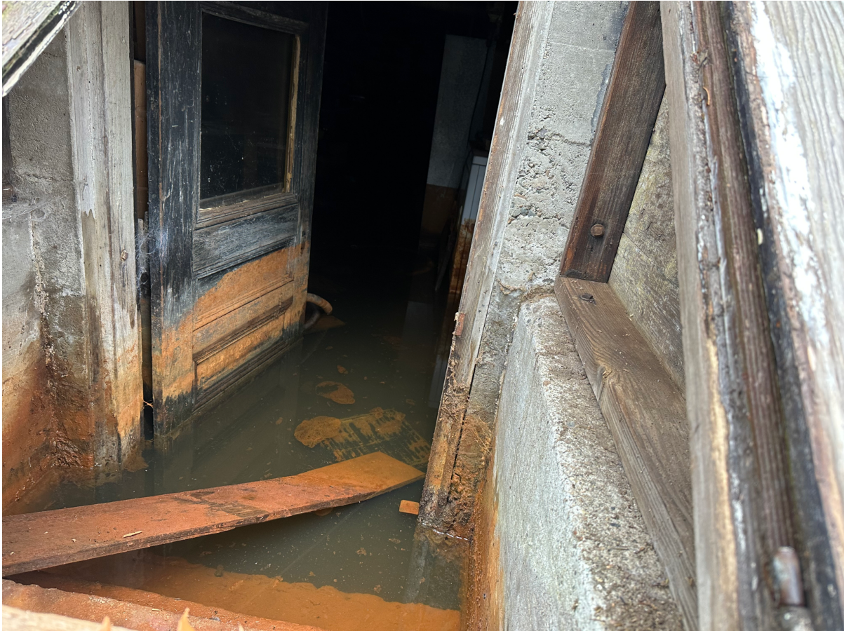
EXHIBIT C Photo of Flooding in House Basement
