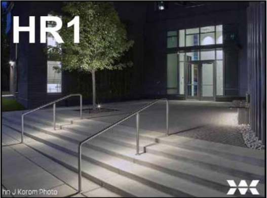
HR1 Stair Lighting Concealed beneath Handrails
