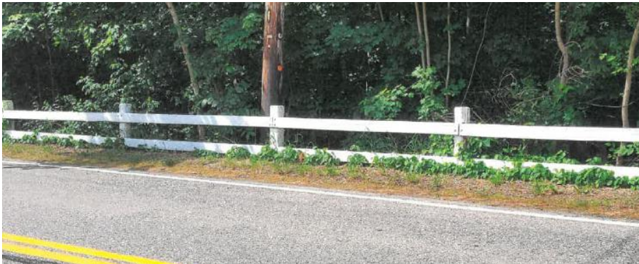
Current guardrail to be replaced at Dedham Ave and Central Ave
