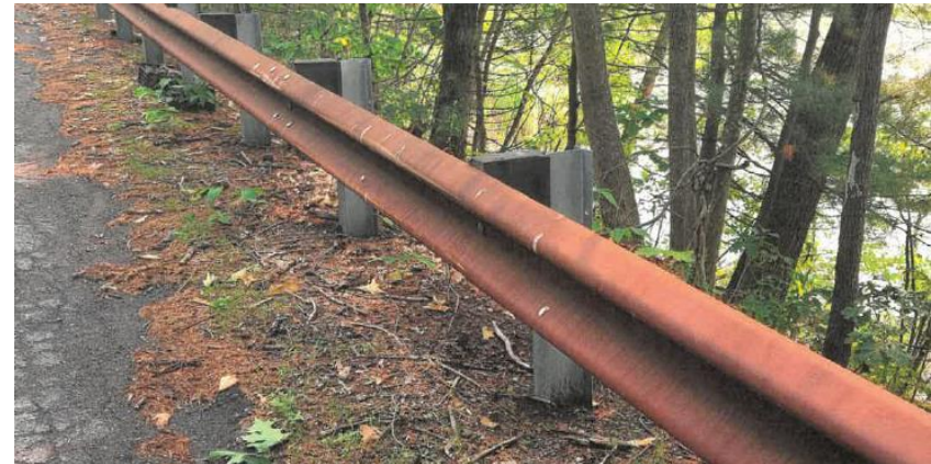
Proposed replacement for high volume roads – Corten Rail with Steel Posts or equivalent
