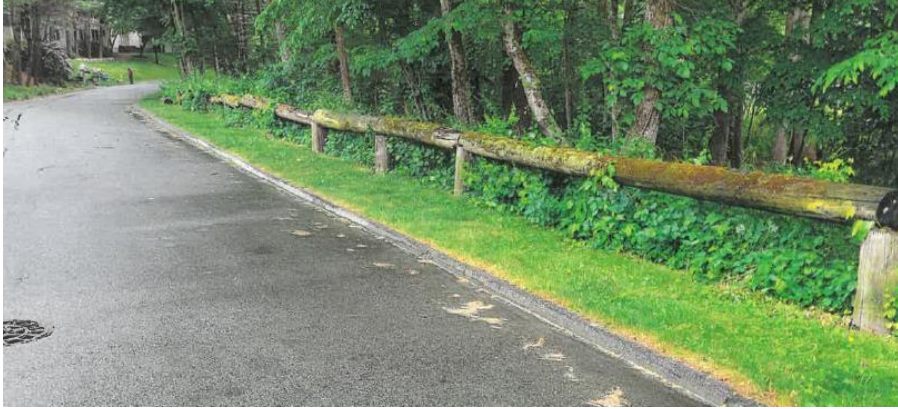
Current guardrail to be replaced at Farley Pond
