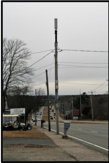
Figure 5D: Verizon Wireless Small Cell site “SC08” near 533 State Rd.
