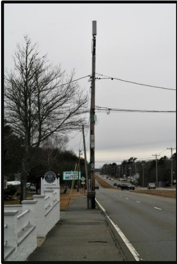
Figure 4C: Verizon Wireless Small Cell site “SC05” near 653 State Rd.
