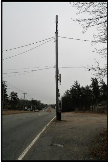
Figure 6E: Verizon Wireless Small Cell site “SC10” near 789 State Rd.
