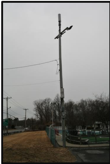
Figure 7F: Verizon Wireless Small Cell site SC11 near 900 State Rd.
