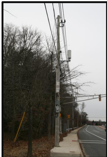
Figure 2A: Verizon Wireless Small Cell site “SC01” near Faunce Corner.
