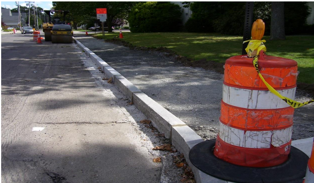
New curb and sidewalk excavation on west side of Dedham Ave. from original project limit to Lincoln St.
