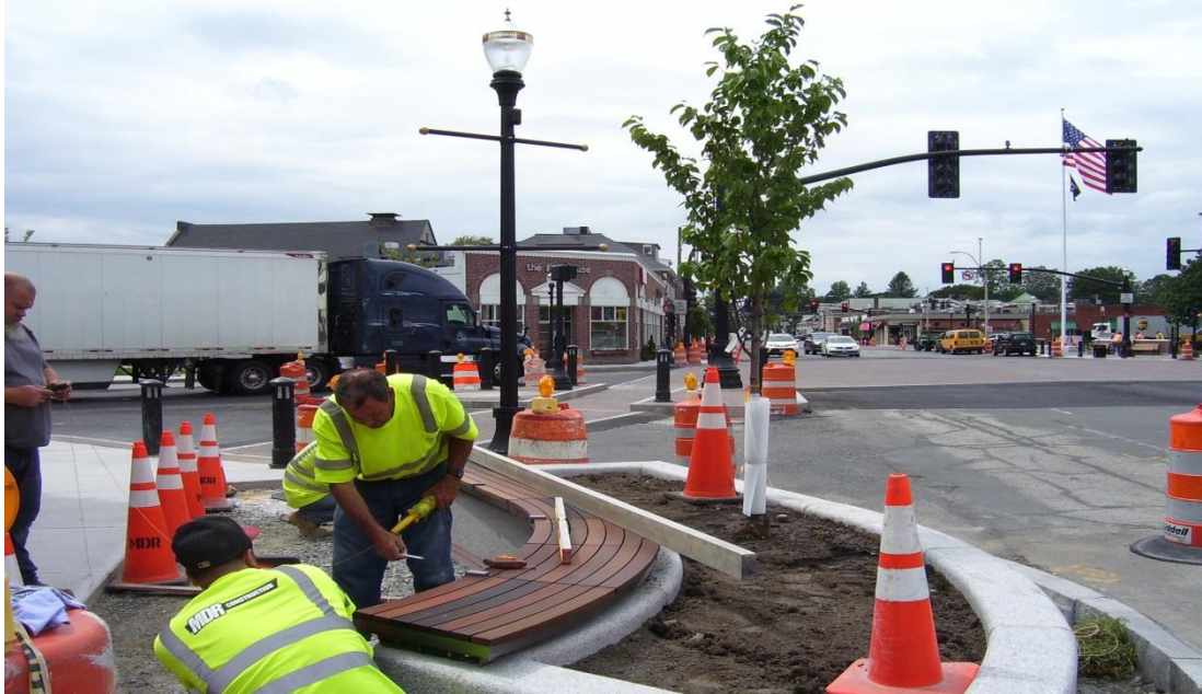
Installing wood seat on granite planter on the southeast corner of Great Plain Ave. and Dedham Ave.
