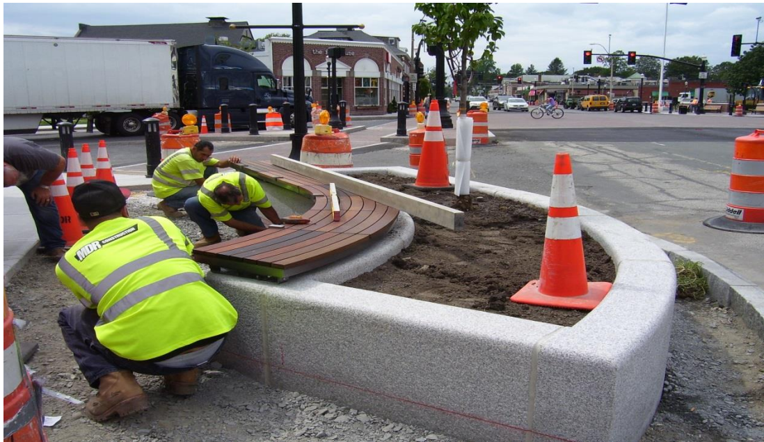
Installing wood seat for granite planter and setting grade for concrete sidewalk
