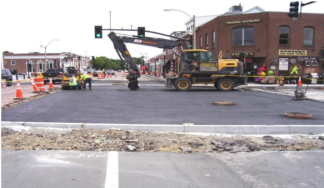
Granite curb being set and asphalt base being installed for brick paver crosswalk in Great Plain Ave. at Chestnut St.
