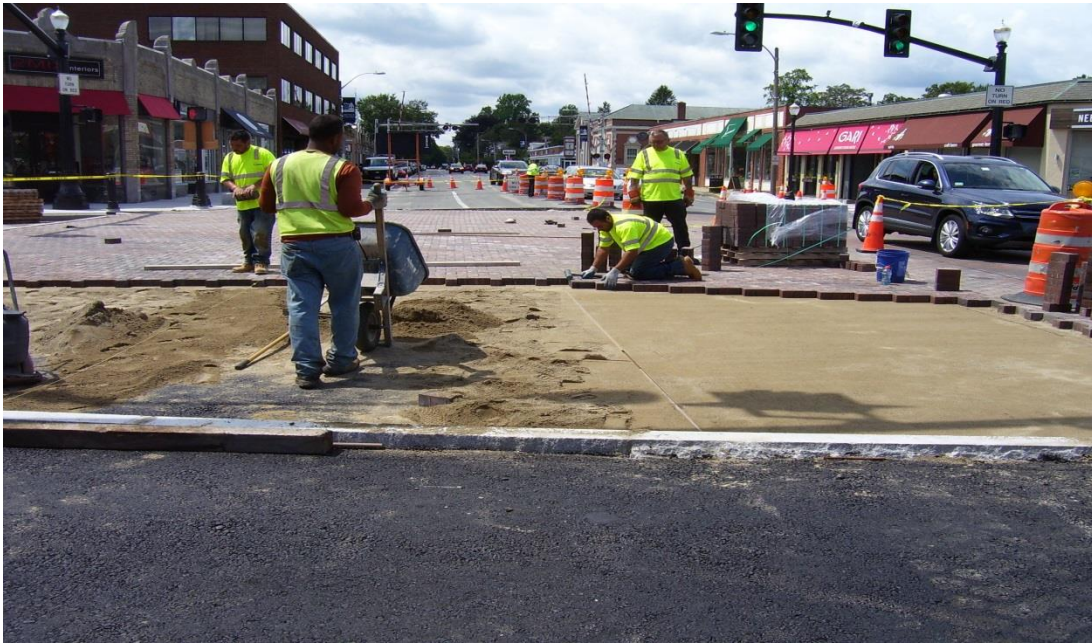
Installing sand bedding and brick pavers in Great Plain Ave. at Chestnut St.
