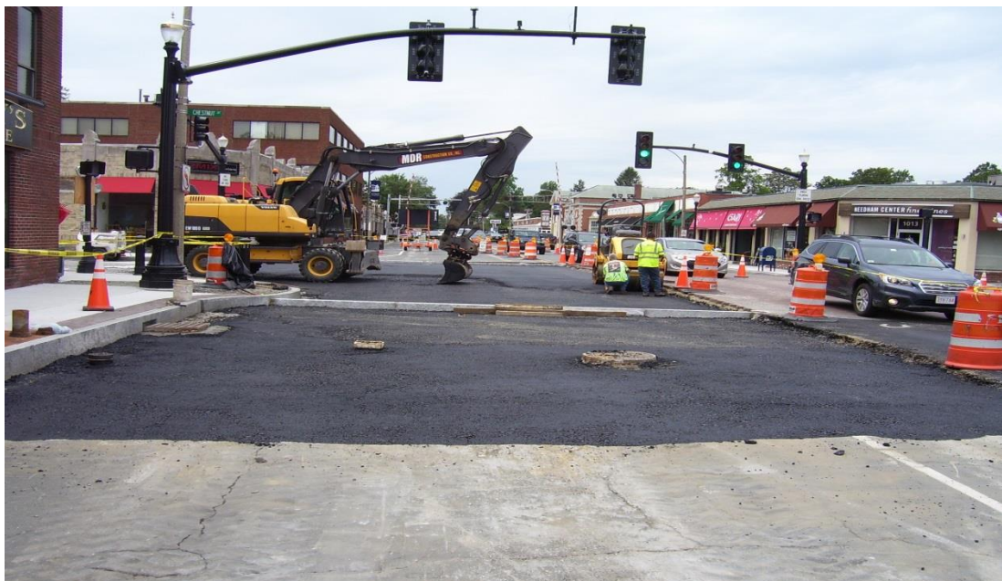
Installing asphalt base for brick paver crosswalk and full depth reconstruction (in foreground) in Great Plain Ave. near Chestnut St.
