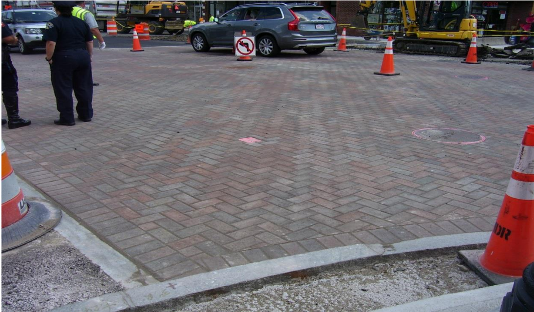
Completed brick paver crosswalk on the north side of Great Plain Ave. at Chapel St.
