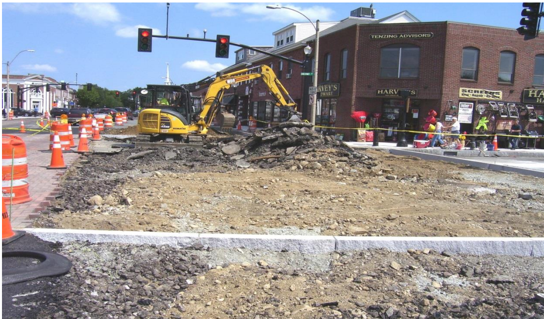
Granite curb installed and excavating for brick paver crosswalk installation in Great Plain Ave. at the intersection of Chestnut St.
