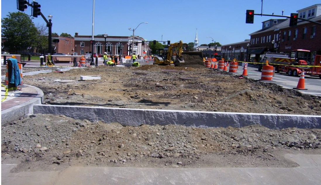
Excavation and setting granite curb for brick paver crosswalk on the north side of Great Plain Ave. at Chapel St.
