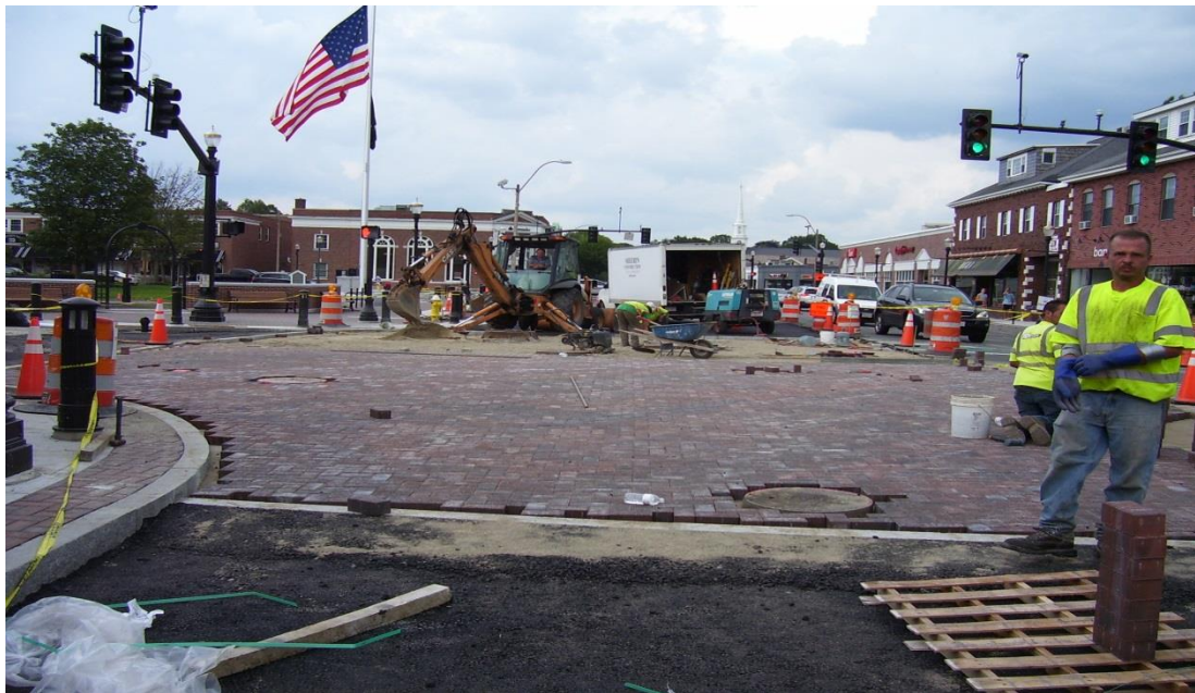
Setting brick pavers and bedding sand in crosswalk at intersection of Great Plain Ave. and Chapel St.
