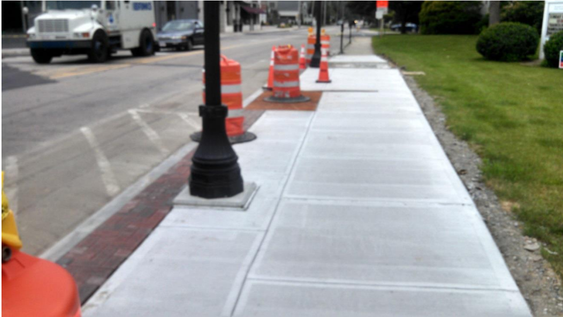
New concrete sidewalk in Dedham Ave. west showing brick paver strip and tree grate
