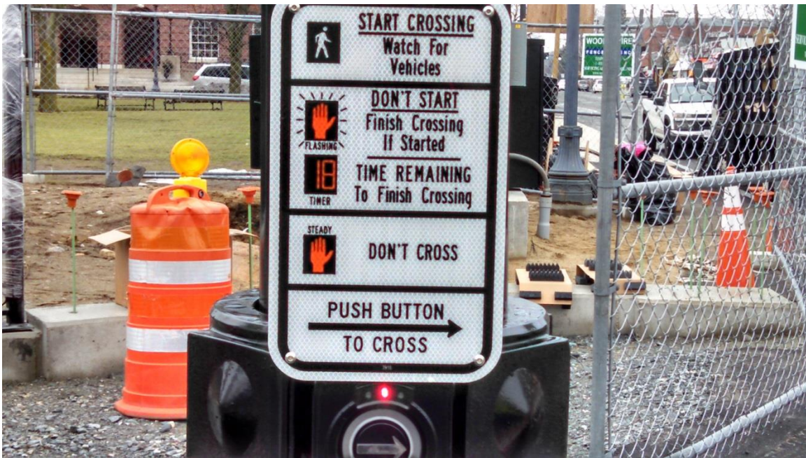
New pedestrian pushbutton in operation at the northwest corner of Highland Ave. and Great Plain Ave.
