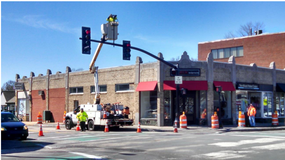
New traffic signals in operation and camera being installed on the southwest corner of Chestnut St. and Great Plain Ave.
