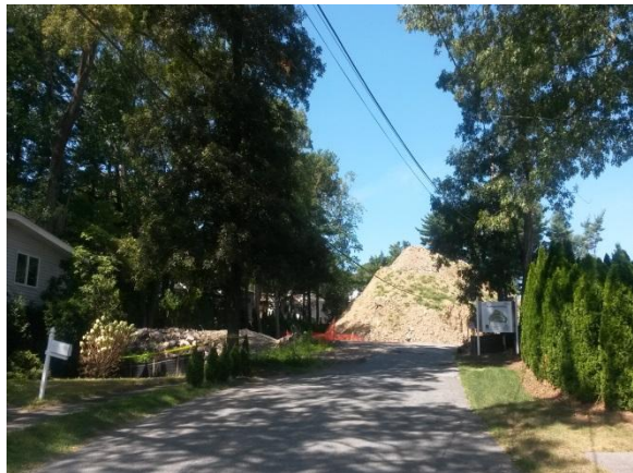
Low hanging fiber optic cable at 30 Rockwood Lane. Sign reinstalled.
