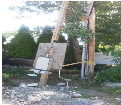
Temporary electric panel installed no connection to power supply
