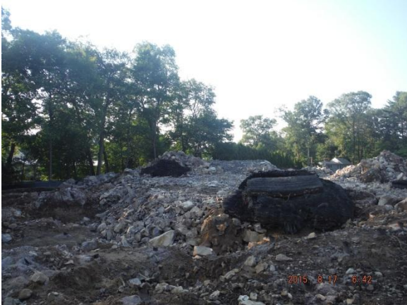
Blasting mats and excavated stockpiled blasted rock. Unsafe depression and unstable material.
