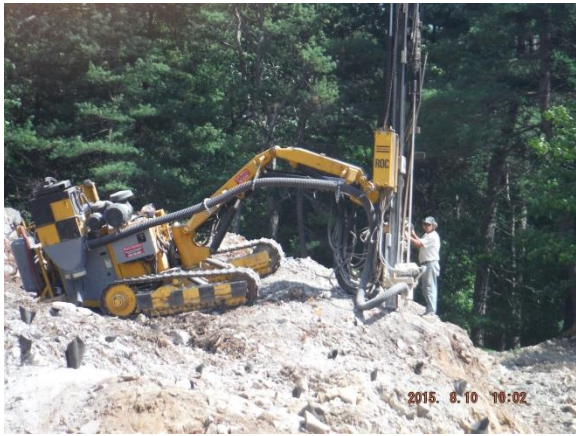
Rock drilling continues in the east central & northeast sections of the site
