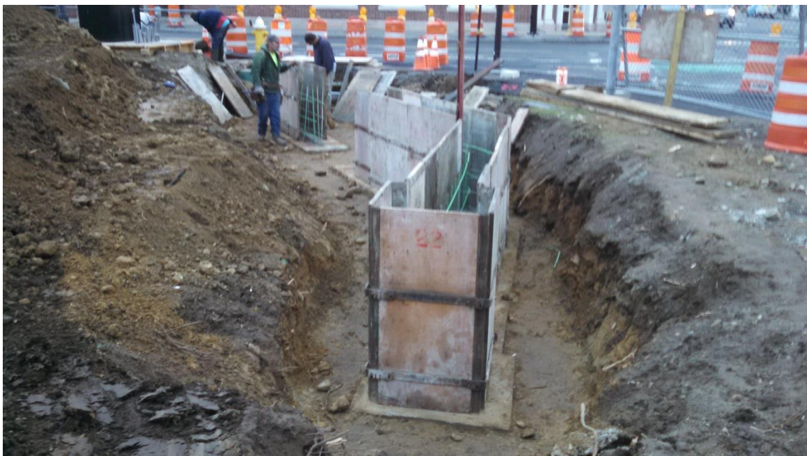
Setting re-bar and forms for the masonry wall foundation on the east side of the Common
