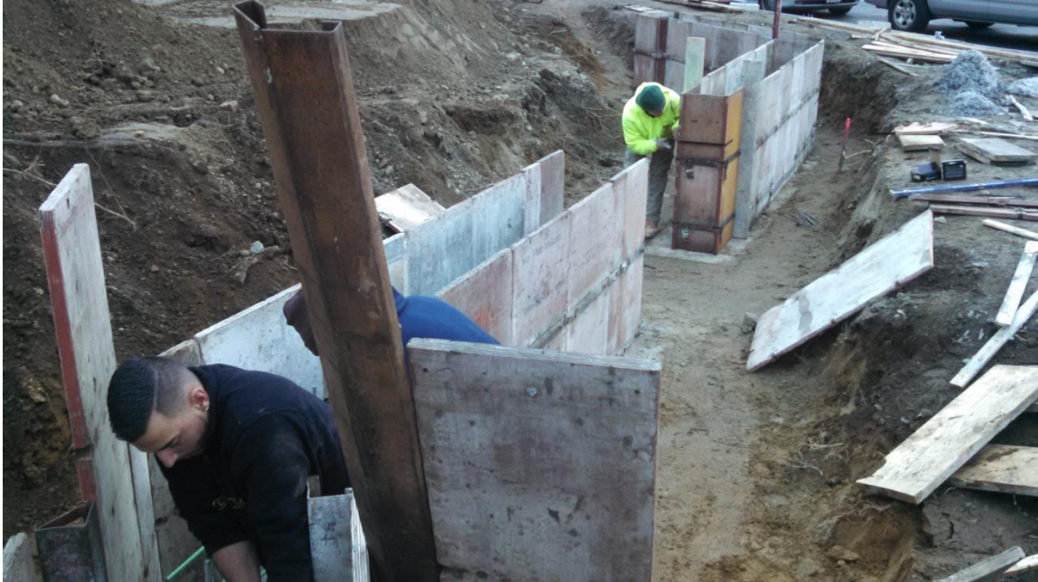
Setting re-bar and forms for the masonry wall foundation on the west side of the Common
