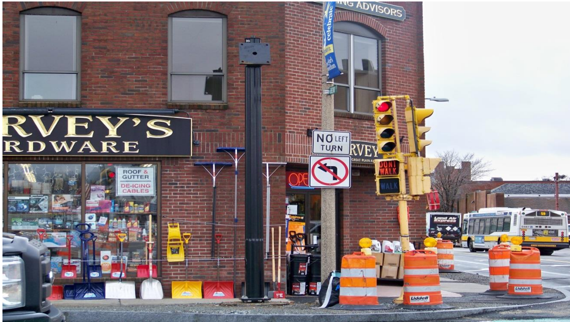
New traffic signal light pole installed on southeast corner of Great Plain Ave and Chestnut St
