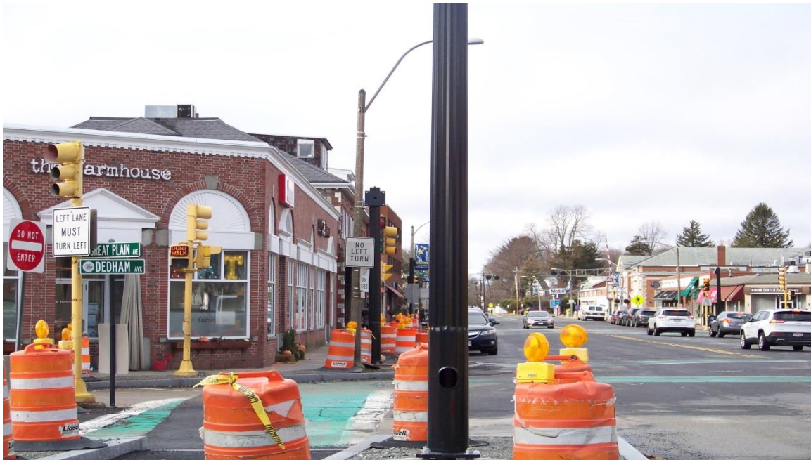
New traffic signal light pole installed on southwest corner of Great Plain Ave and Dedham Ave (background) and in new island at intersection of Great Plain Ave. and Dedham Ave. (foreground)
