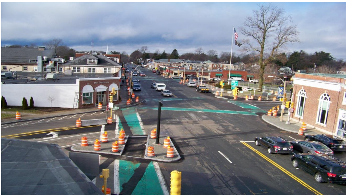
Photo of overall project status from easterly limit of project looking west
